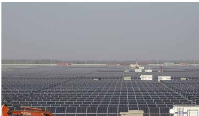
Fig. 5. The 100 MW Quaid-e-Azam Solar Park, Bahawalpur, Pakistan [14].
