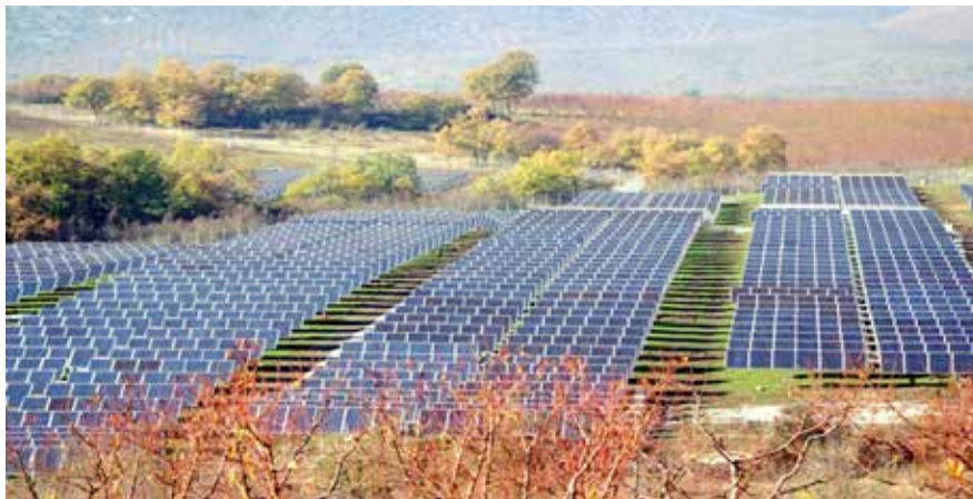
Fig. 6. The 8 MW PV plant using horizontal single axis solar tracker in Greece [16].
