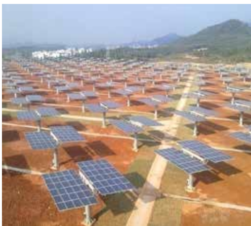
Fig. 7(a). The TTDAT PV power plant [16].
